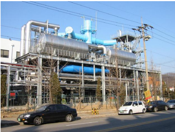
Solvent Recovery Plant in South Korea
